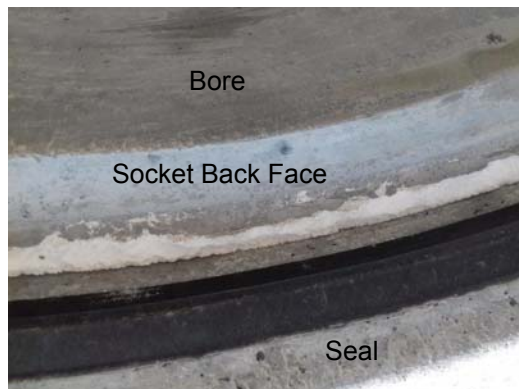
Fig. 1 Residual polystyrene in back corner of socket.
