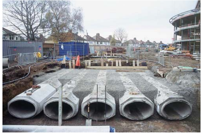
The polygonal profile provides a structurally efficient drainage solution for shallow culverts under highways
