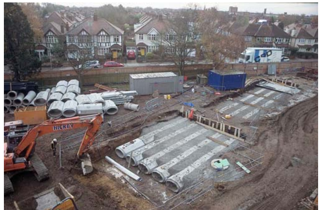
Compaction of backfill is required only to prevent surface settlement. Special backfill materials are rarely required
